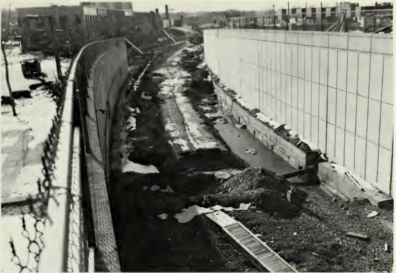
DEPRESSED ROADBED and retaining walls are under construction on the Braintree Extension just south of Quincy Center Station.
